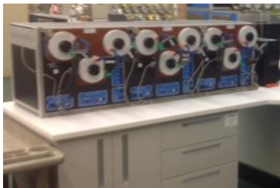
Figure 5 Three position WECO 2350 Test Boards – Testing nine Smart Light Modules simultaneously. 2
